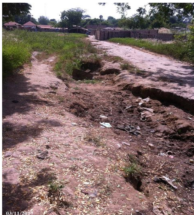
Figure 2 Road condition in Kaba kama taken 03/11/2017
